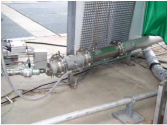
Fig. 26. Heat-wire-measurement, prior to the system the motor driven valve with battleship-actuator.
